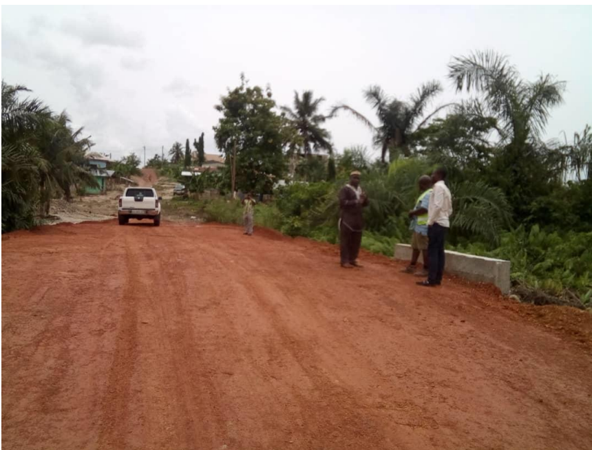
CONST. OF 2 NO. 2/1200 MM PIPE CULVERT AT ASANKRANGWA NEW MARKET & ASANKRANGWA-YIREHO ROAD-COMPLETED
