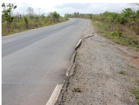
Edge damage on central corridor in Togo
