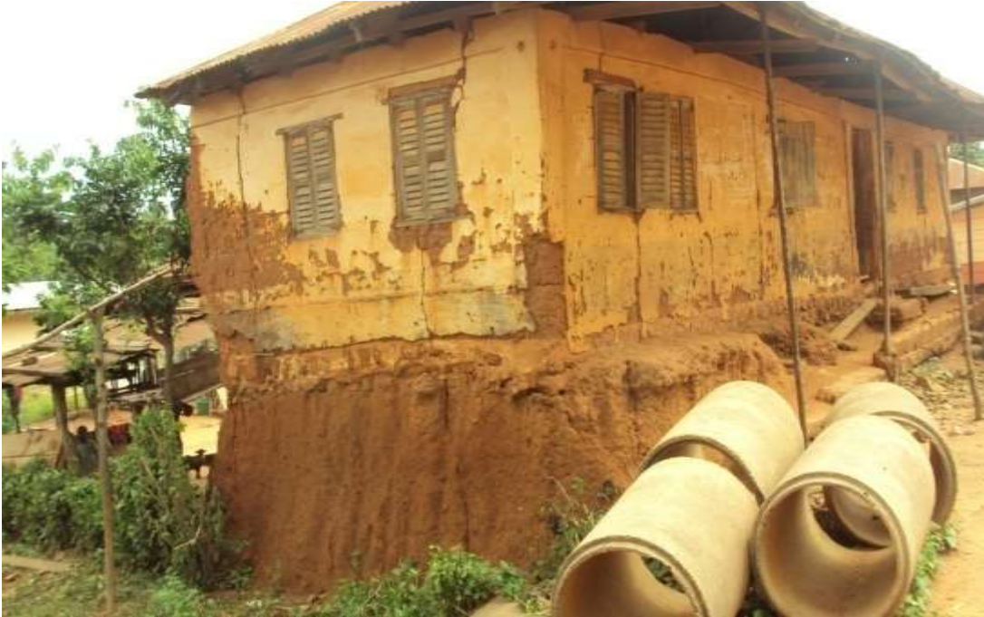
Figure 1.14: Erosion along residential buildings (exposed foundation) in Nkonya Tayi
