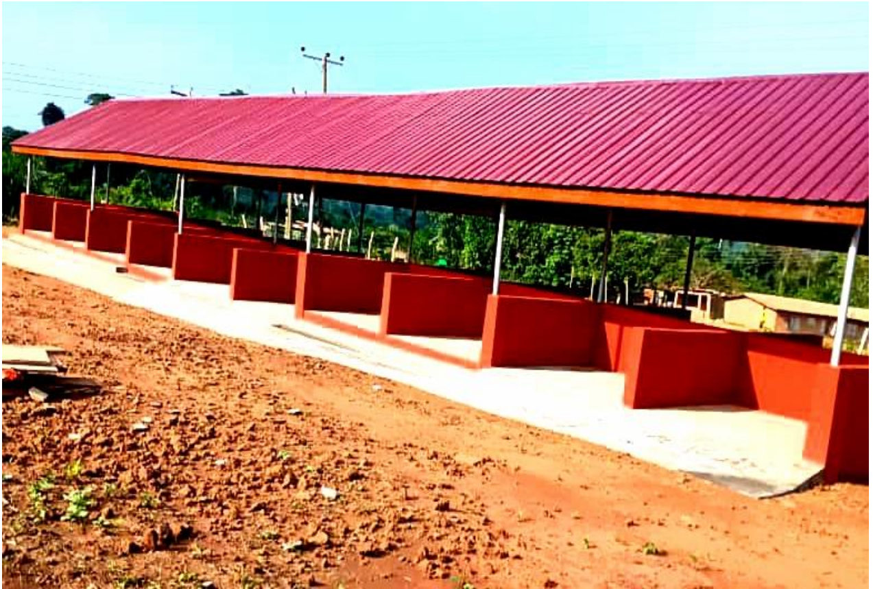
CONSTRUCTION OF 20 UNIT MARKET SHED WITH 4 UNIT WC TOILETS AT BOWIRI AMANFROM
