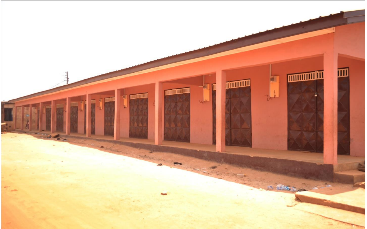
CONSTRUCTION OF 10 UNIT MARKET STORES WITH 4 UNIT WC TOILET FACILITIES AT KWAMEKROM MARKET
