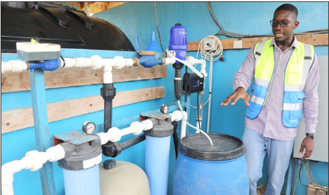
Sylvester Adjapong director of impact and quality for Access Development explains the Nexus purification system at Sekyere Aboaboso in Wassa East
