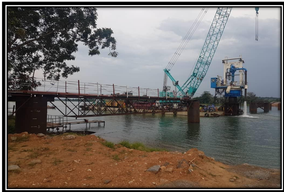
Construction of Rail Bridge (Viaduct) across Volta River Between Senchi and Old Akrade
