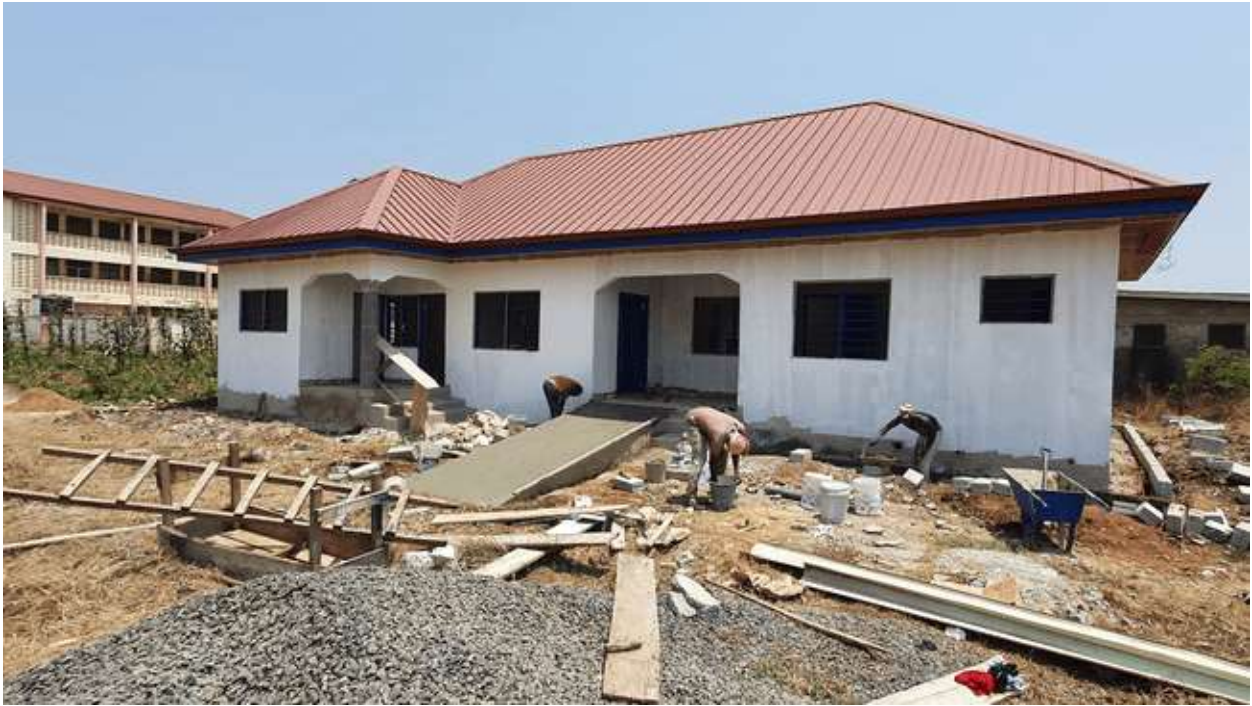
Construction of Sickbay At Tetteh Ocloo School for the Deaf Adjei Kojo
