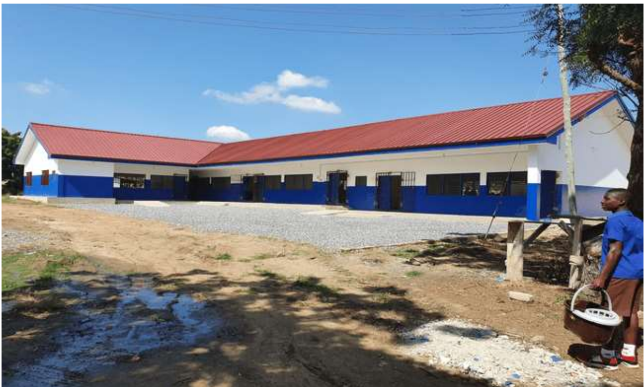
Construction of Single Storey Vocational Training Centre At Tetteh Ocloo School for The Deaf Adjei Kojo
