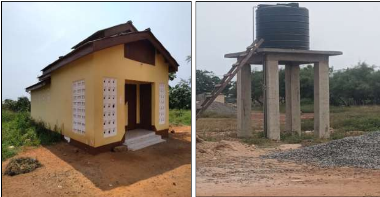
Connection of Water and improvement of Sanitation facilities (Toilets) at Prampram and Old Ningo Markets
