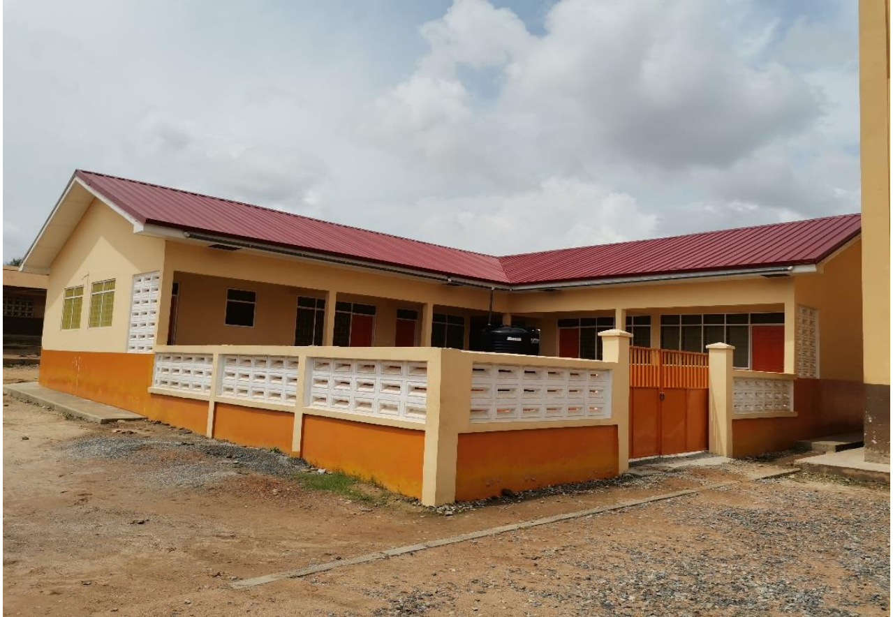
Construction of 1 No. 2 Unit KG Classroom Block at Ofankor M/A Basic School
