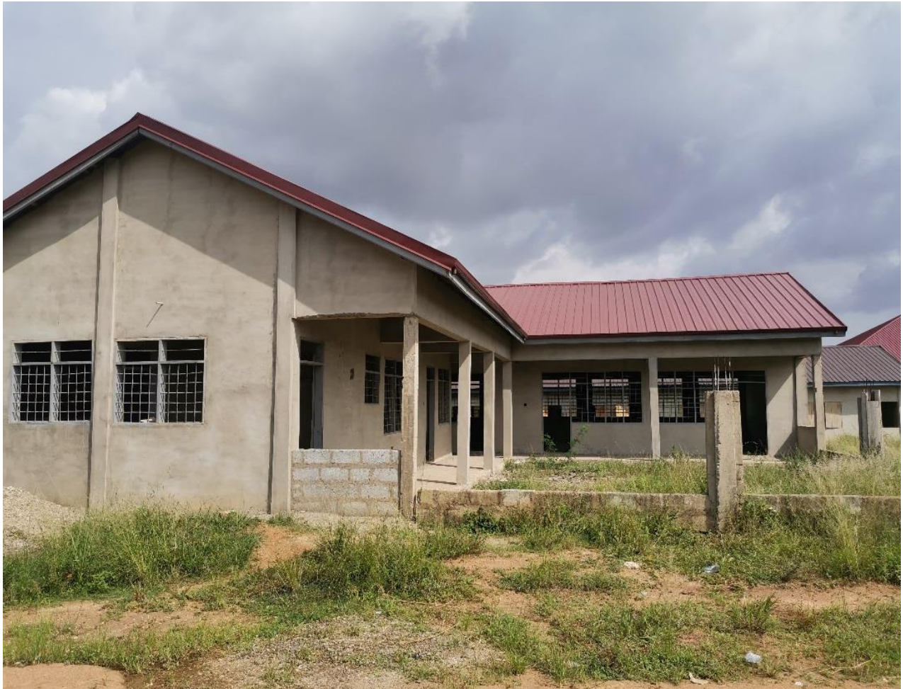
Construction of 1 No. 2 Unit KG school block for the Presbyterian Basic School at Afiaman
