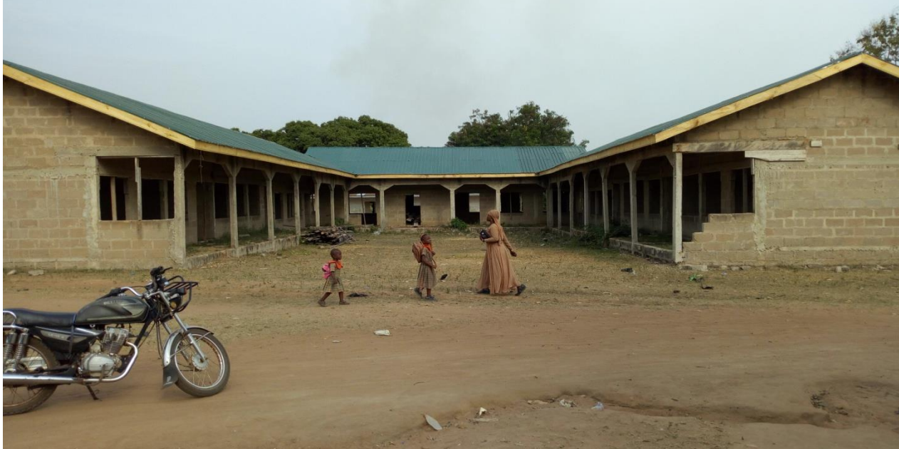
Construction of 1No.6-Unit Classroom Block, Office, Store, Computer laboratory and Staff Common Room with 1No. 4-Seater KVIP Toilet at Hwidiem Presby Primary
