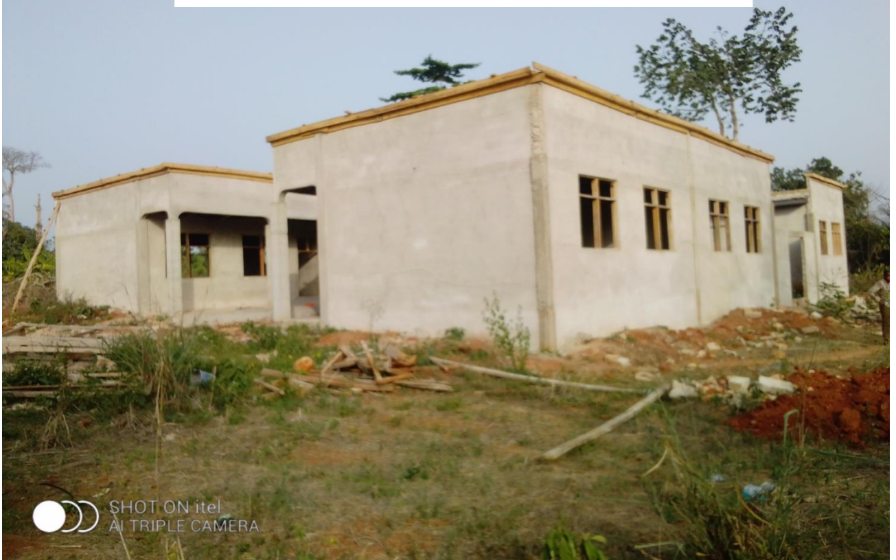
Construction of 1No. 3-Unit Classroom Block with 3 Bedroom Dormitory Accommodation at Dadiesoaba Girls Model School
