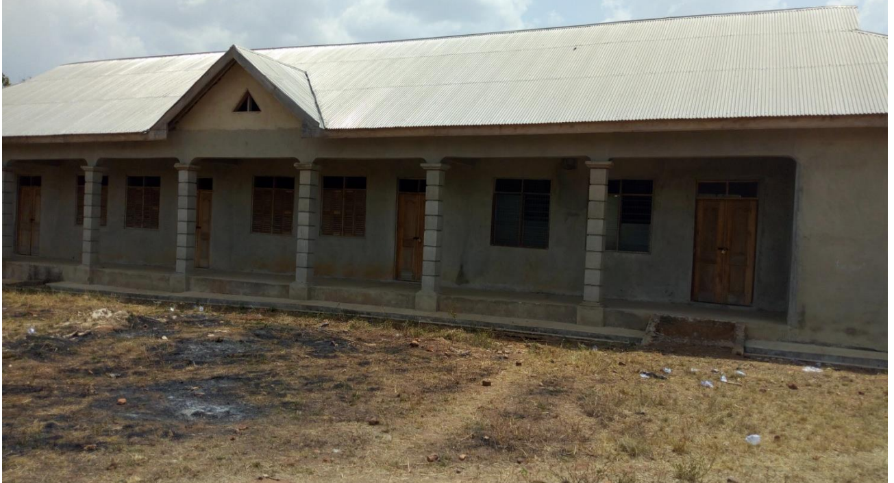
Construction of 1No. 3-Unit Classroom Block with Office, Store, Computer Lab and 2-Seater Toilet Facility at Mehame (DACF Project)
