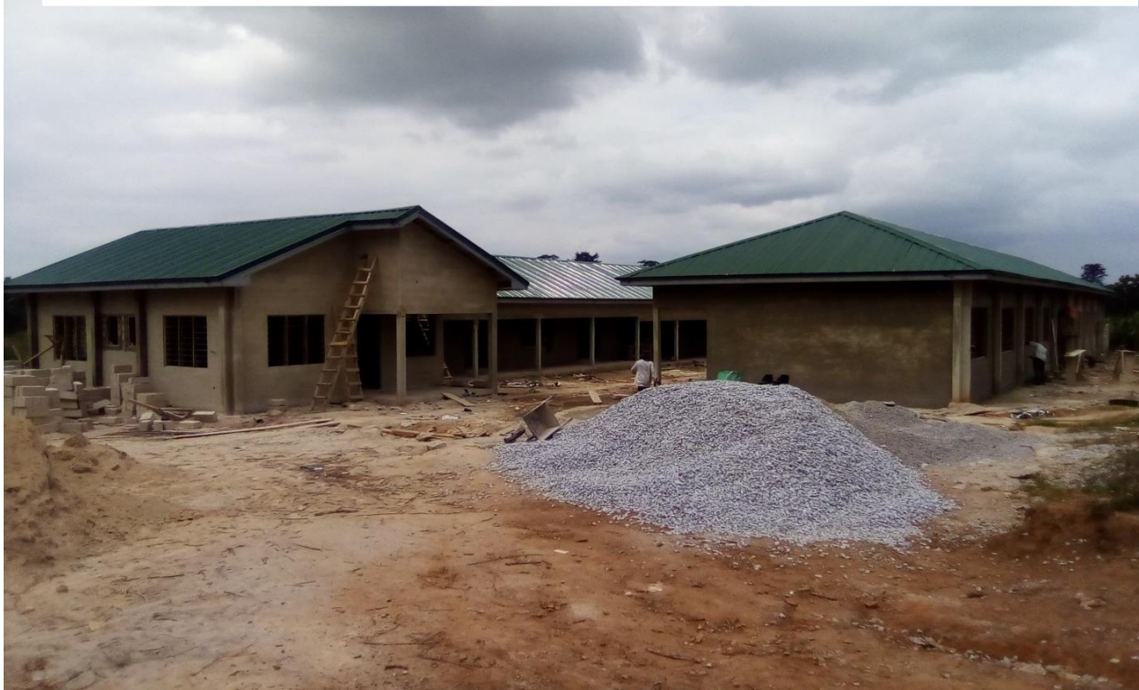
Construction of 1No.12-Unit Dormitory for Girls at Hwidiem SHS (Middle Belt Authority)
