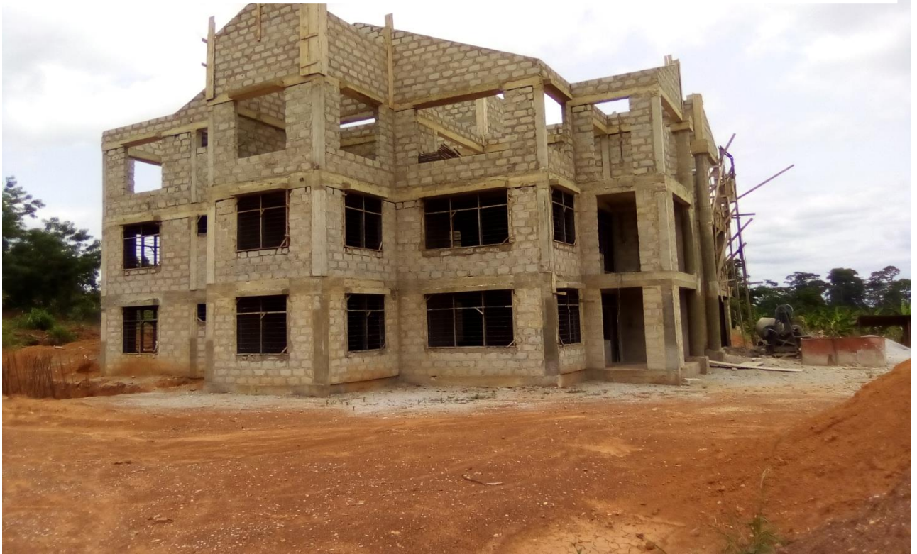
Construction of 1No.3-Unit Classroom Block with Ancillary Facilities at Acherensua SHS (GETFund)
