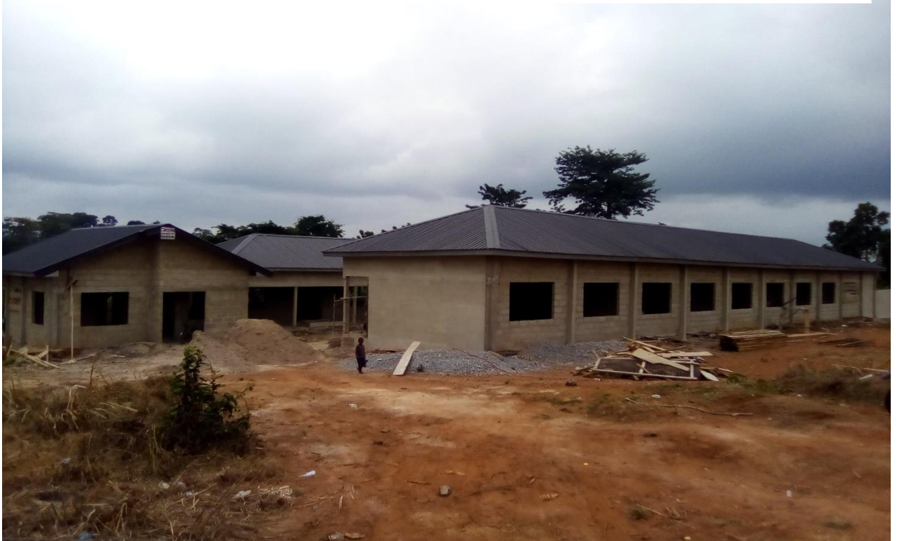
Construction of 1No.12-Unit Dormitory for Girls at Acherensua SHS (Middle Belt Authority)
